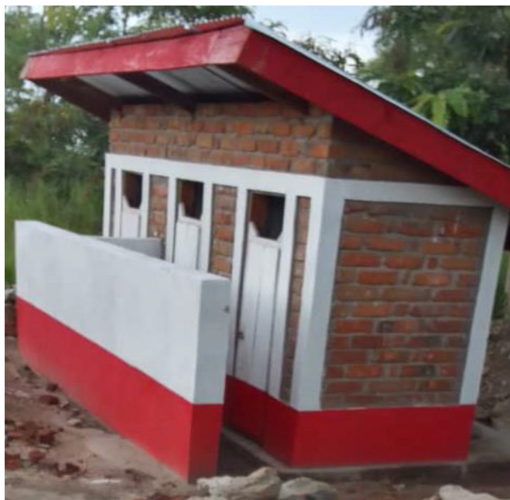
Latrine constructed as part of school construction work in EP Hakima in Fizi
